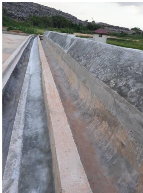
Figure 7: Headworks for faecal sludge discharging at Oti
